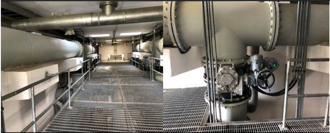
Pumping system for the back flushing and filtration to control head losses
